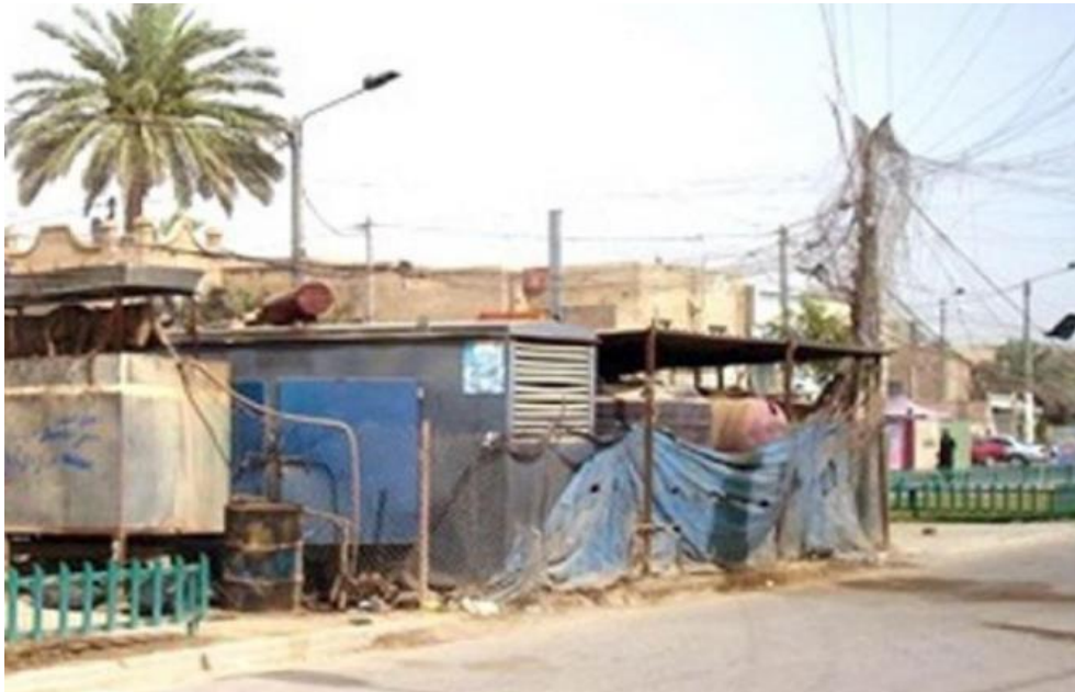
Figure 1: private diesel grid [8].
